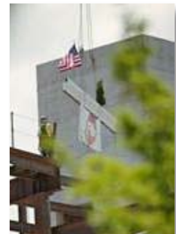
Signed steel beam being put into place at the top of the Utah Valley Convention Center
